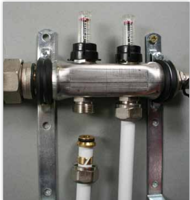
Pipe to Manifold Connection
